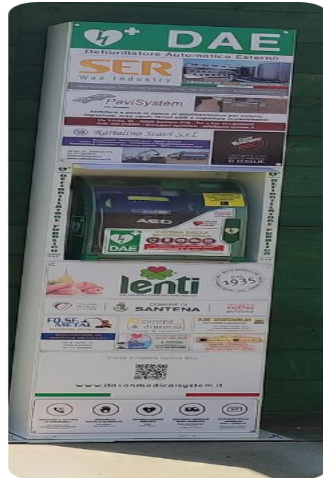
Public defibrillator installation for community safety
